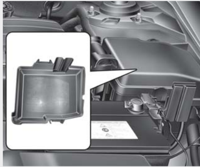
Engine compartment fuse panel
