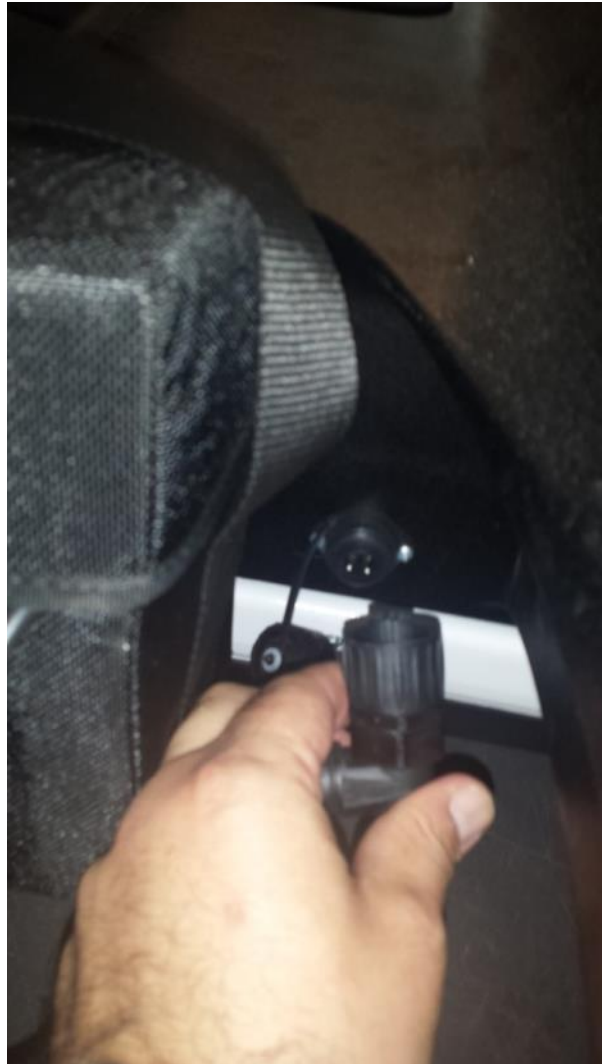
Fig. 4.14 – connectors of the electric engine batteries
