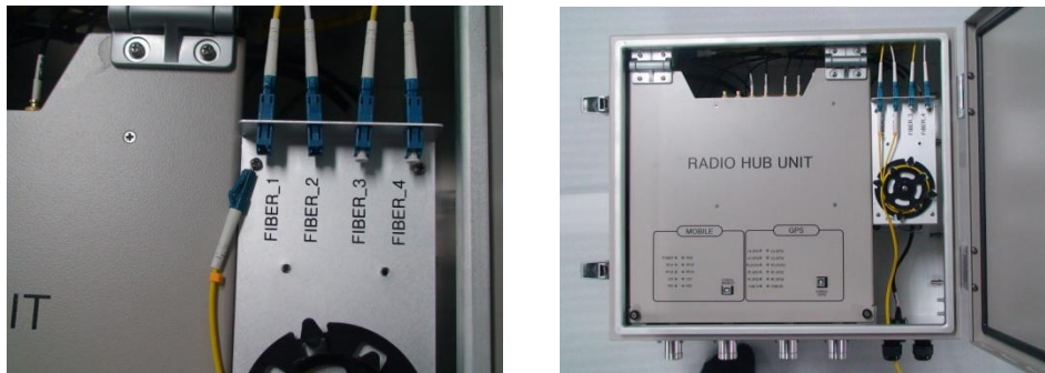
Figure 3-9 Fiber cable connection on RHU
