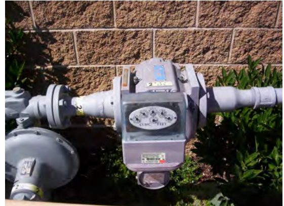
Sensus commercial ERT Module mounted on a Dresser meter with an instrument drive
