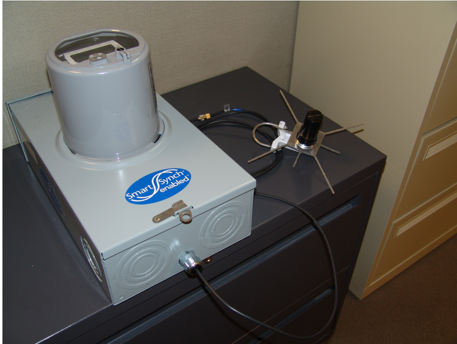
FIGURE 2 Typical routing of SSI Monopole cable for external remote antenna.
