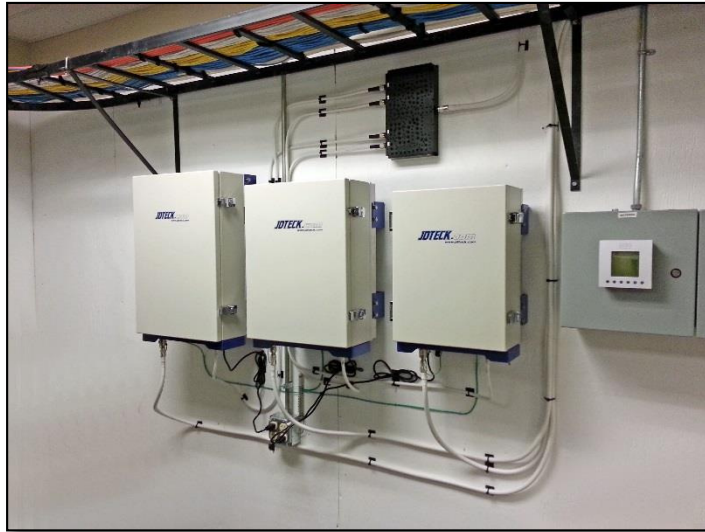
Example of repeaters installed in communications closet.
