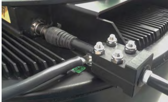
Example of a cable installed in the cable bracket assembly
