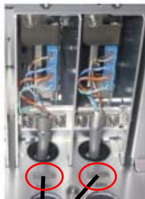
Holes for surge box cover
