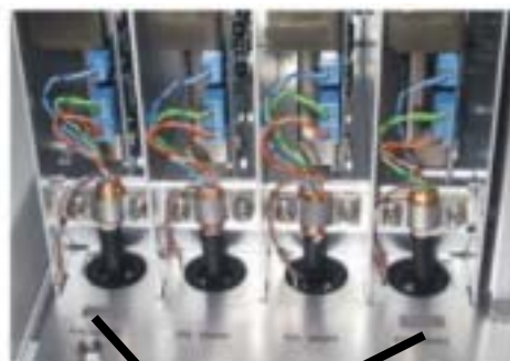
Holes for surge box cover
