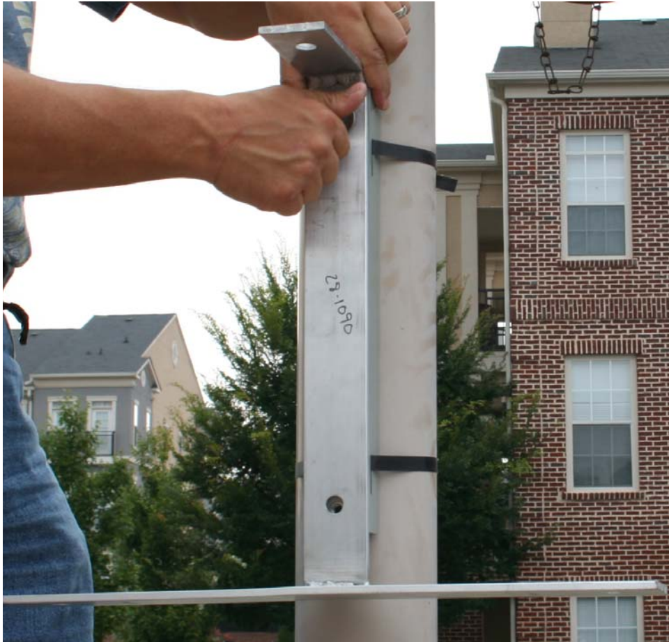
Figure 4 - 5. Antenna light pole bracket attached to mounting bracket
