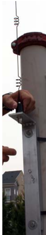
Figure 4 - 7. Connecting the WAN antenna
