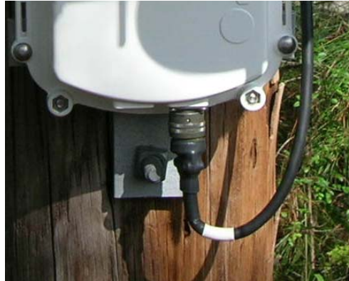
Figure 4 - 1. Cable with drip loop
