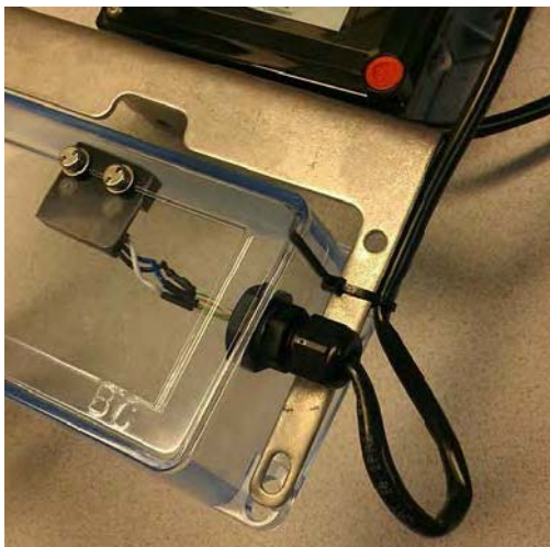
Figure 6 - 18. Switch Cover and GPR Assembly, with drip loop
