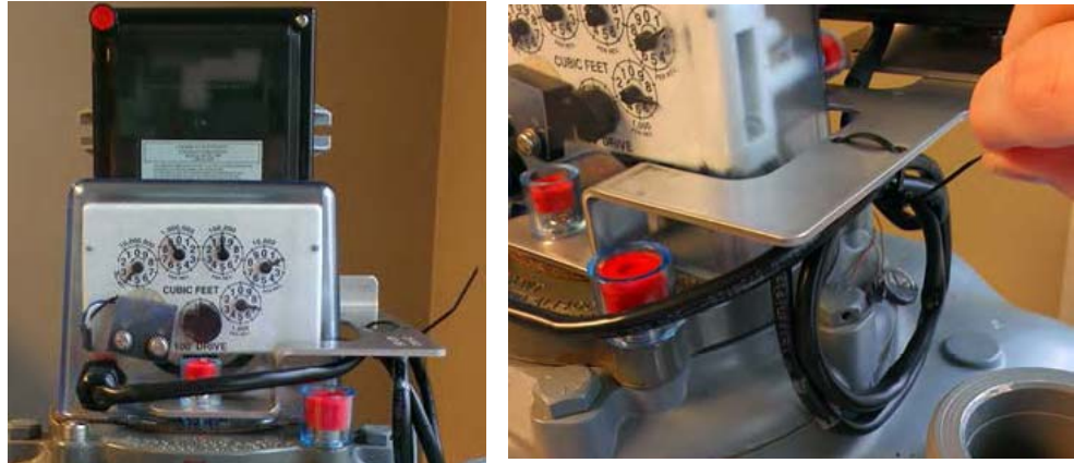
Figure 3 - 28. GPR at Center Rear - Using 28-1441 Bracket
