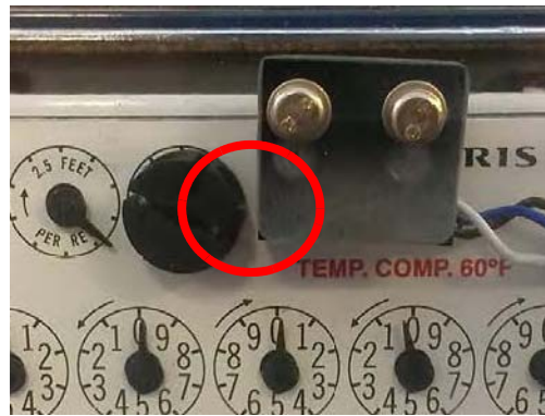
Figure 5 - 24. Gap Must Be Visible Between Wheel and Switch
