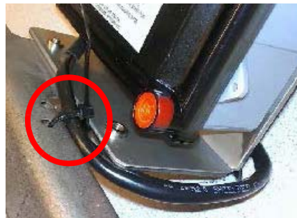
Figure 5 - 20. Excess Coiled Cable Attached Beneath GPR Bracket
