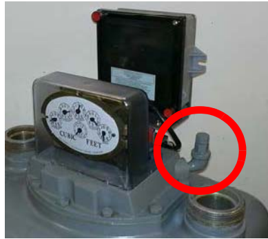
Figure 3 - 13. Meter Pressure Tap
