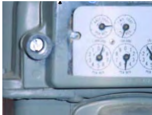
Figure 5.39 Lancaster/National: Meter non-retrofittable
