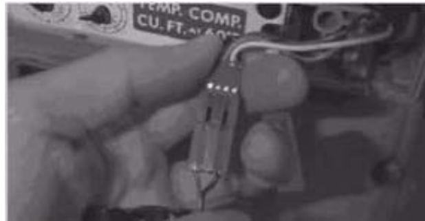
Figure 5.9 American: Connecting the battery
