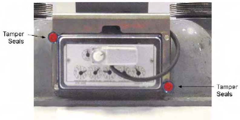
Figure 6.24 Sprague/Actaris: installed tamper seals
