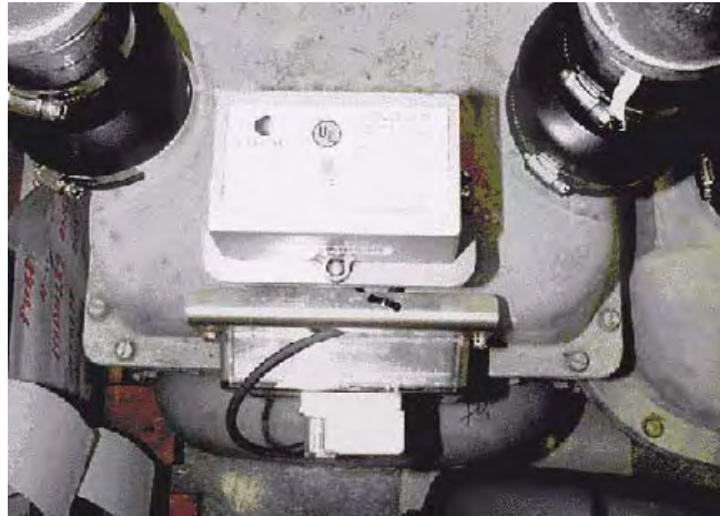
Figure 6.25 Sprague/Actaris: meter with module installed
