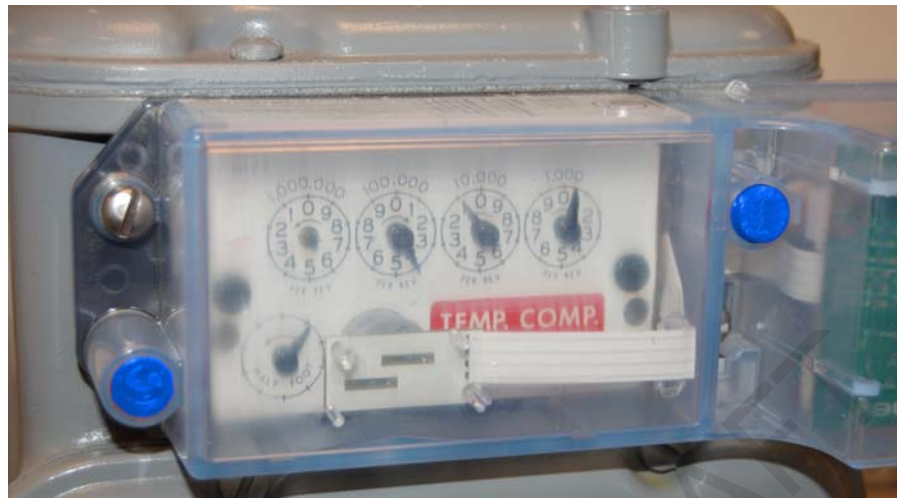
Figure 5 - 16. Meter module with security seals installed
