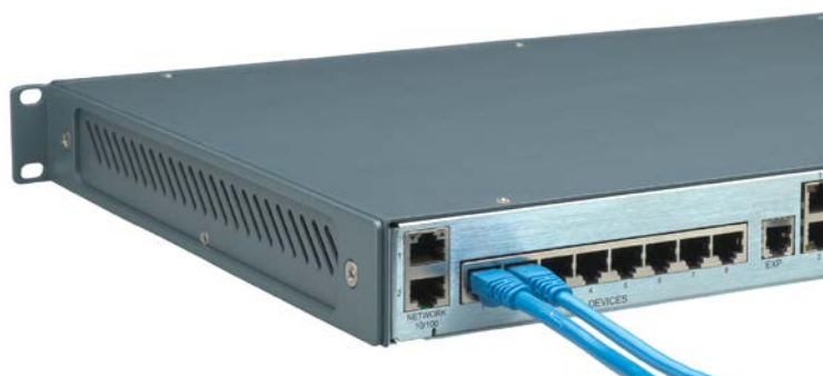
Figure 2-3. Device Port Connections
