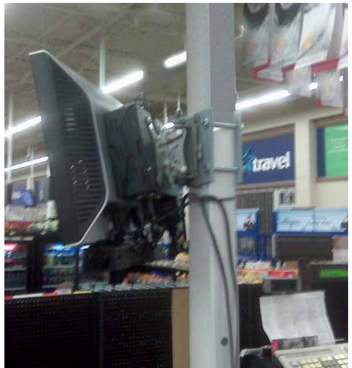
Qtrac Monitor mounted to existing in-store pillar
