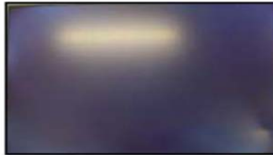
Fuse Open, Abnormal power section
