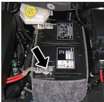
Positive Battery Post
