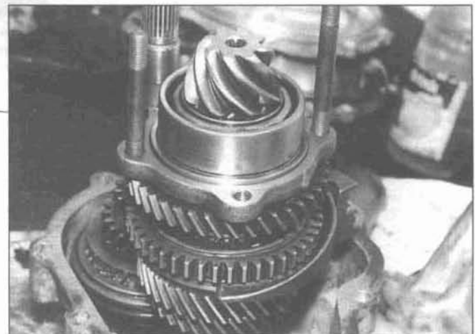
9.77 Install a pair of three-inch long studs in the pinion bearing flange to help you line up the bolt holes (you can't move the flange when it's in position)
