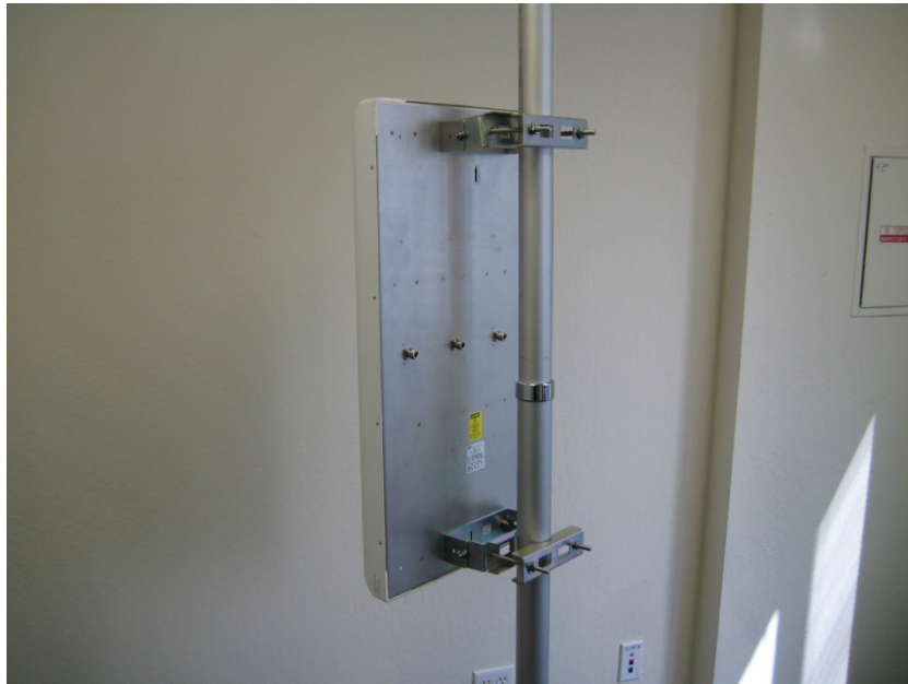
Figure 20 - Base Station Antenna
