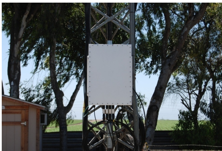
Figure 7 - Pole Mounted Quantum 1000 Base Station Sector
