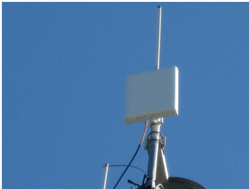
Figure 21 – Typical Antenna Deployment
