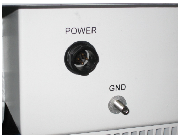
Figure 15 - Base Station Power Input Connector
