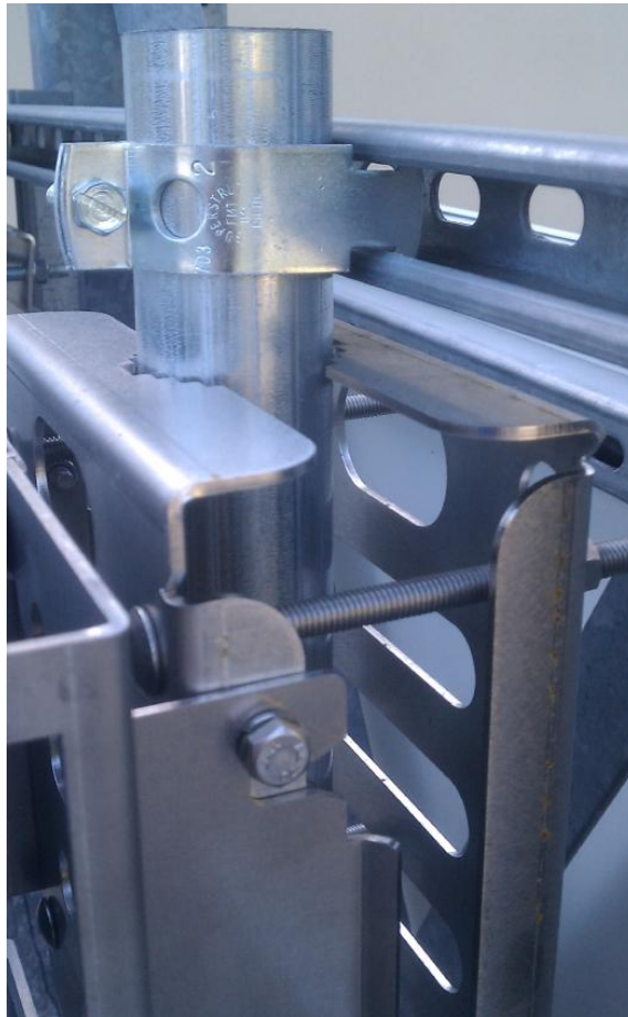
Figure 6: Example Deployment Consisting of Pole Attached to a Metal Frame
