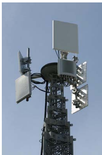
Figure 2: PureWave Quantum 6600 Base Station Mounted on a Tower
