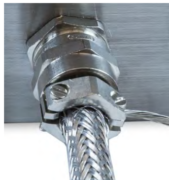
Figure 2-47: Cable and Cable Gland Installed in Enclosure
