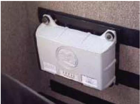
Mounted to the wall
