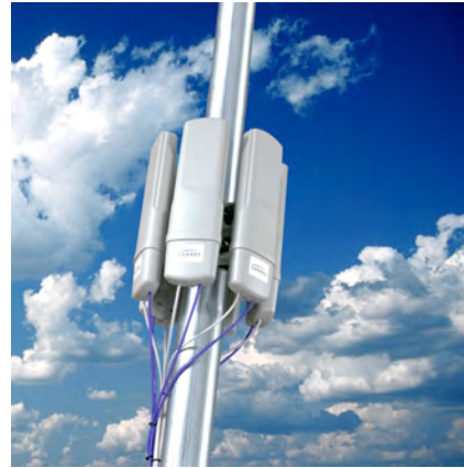
Figure 2: Pole-mounted AP cluster
