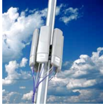
Figure 2: Pole-mounted AP cluster
