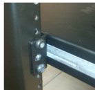
Figure 1b: Rack installation
