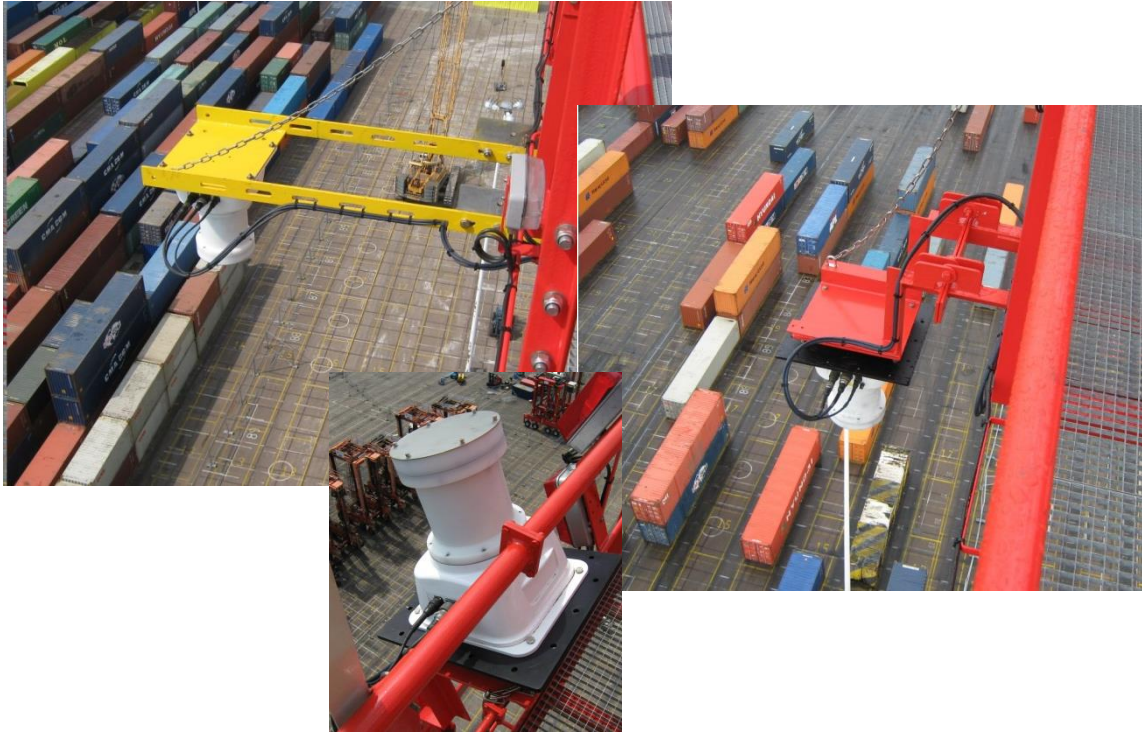
Figure 20 I-200 mounted on a ship to shore container crane. Shown in the deployed position (above) on 2 different bracket arrangements and recovered for maintenance (below)
