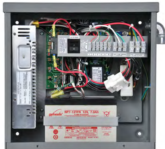
Figure 36 – Outdoor UPS (Cover Removed)
