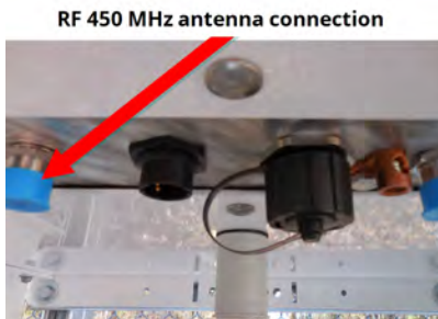
Figure 7 – RF 450 MHz Antenna Connection
