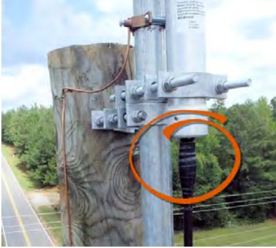
Figure 57 – Weatherizing the RF Antenna Connection
