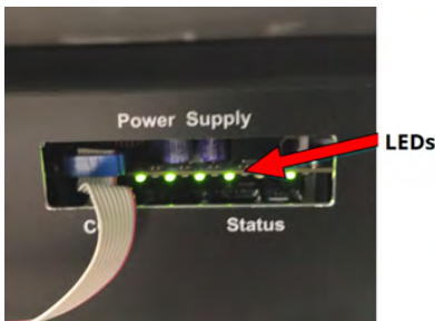
Figure 46 – RMDC Power Supply
