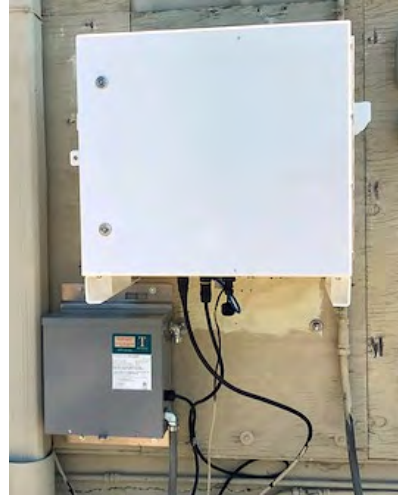
Figure 18 – RMDC Mounted on Wall
