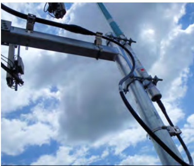
Figure 56 – RF 450 MHz Antenna Connection
