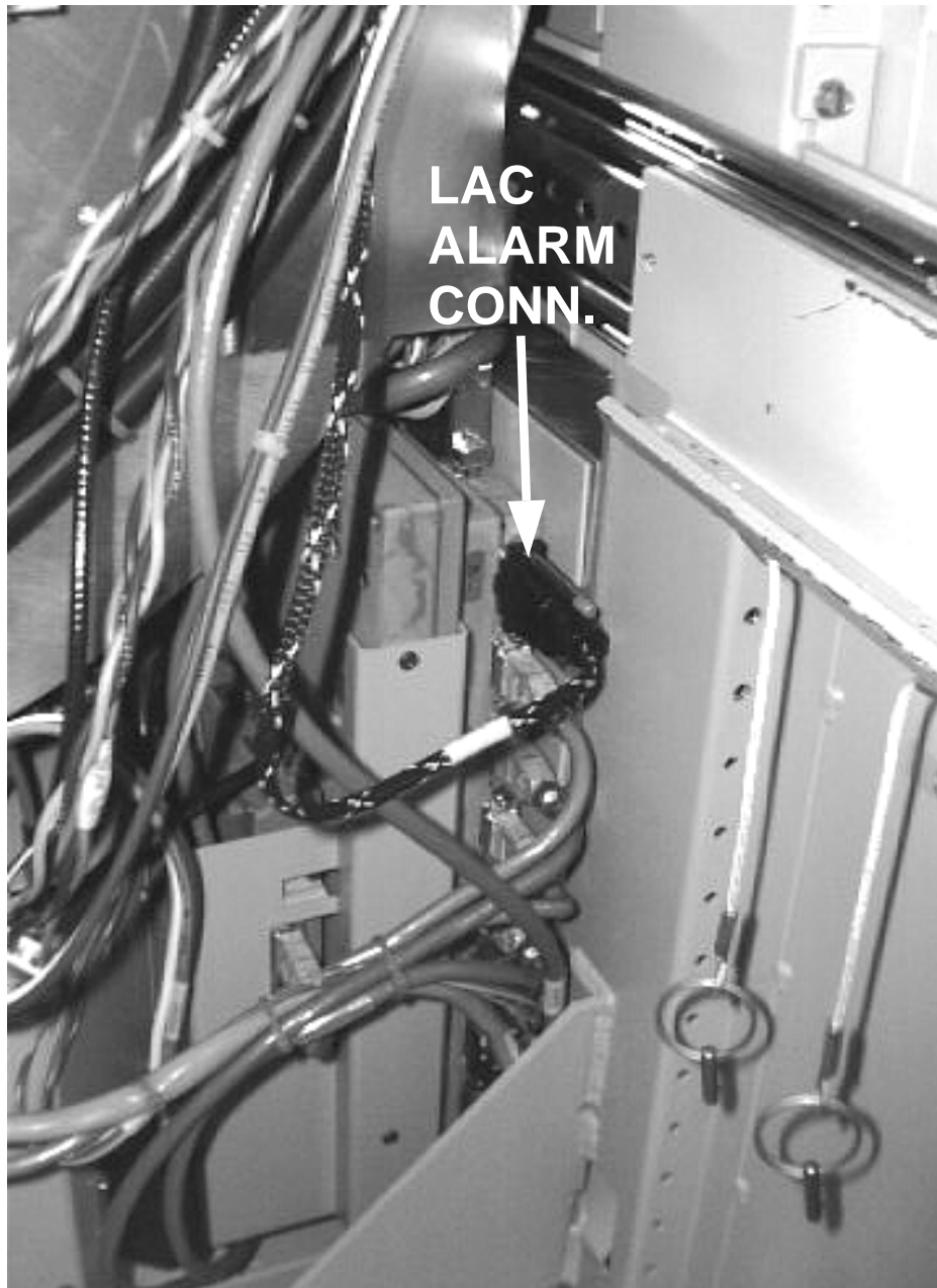
Figure 22-9. Location of the LAC Alarm Cable Connector
