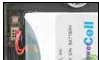
Battery Cable Plugged In
