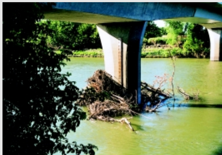
River with debris
