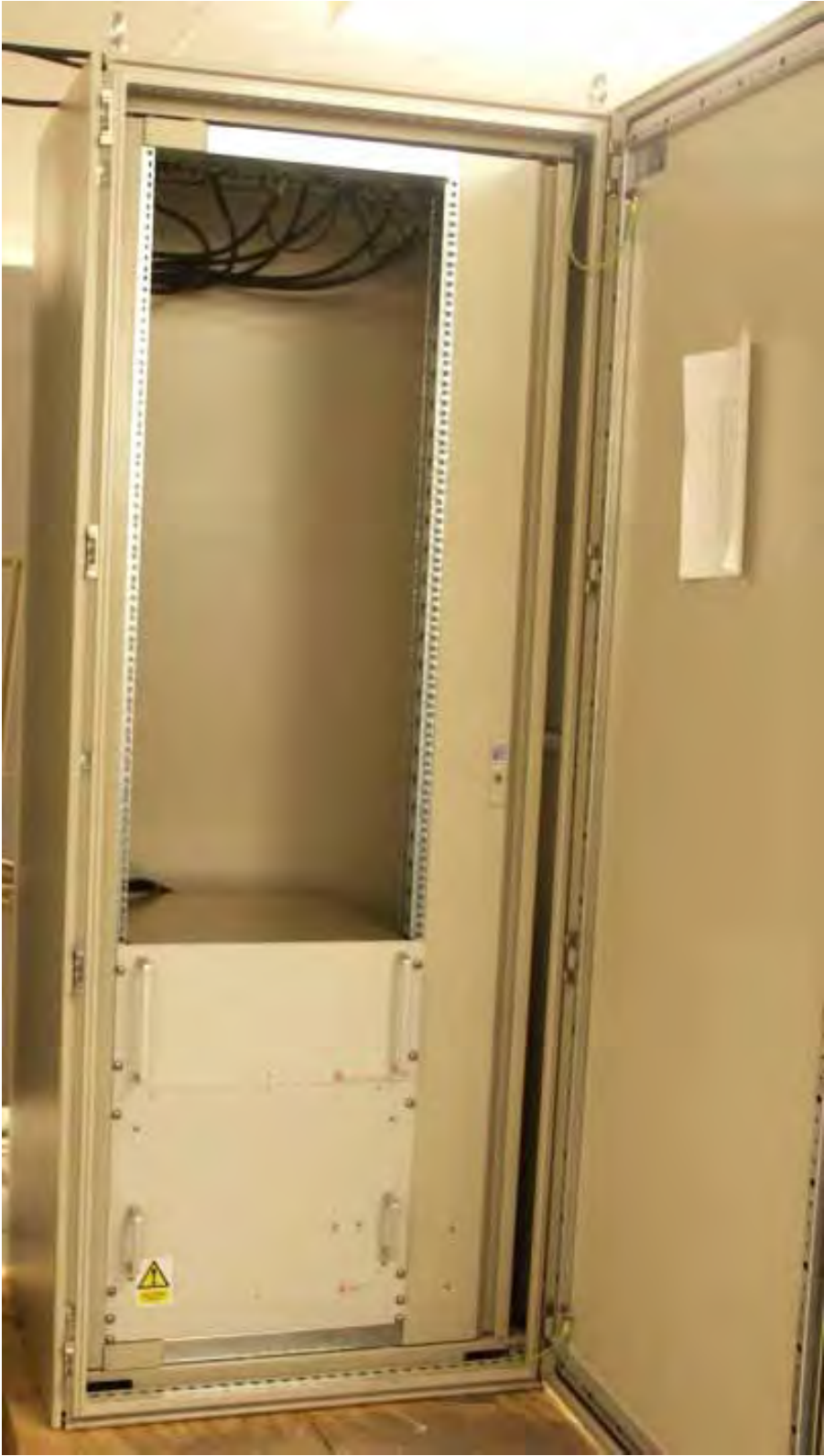
VHF channel modules and amplifier shelves (front view, door open)
