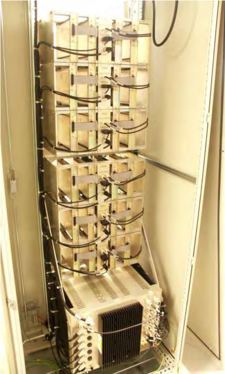
VHF rack (rear view, door open)
