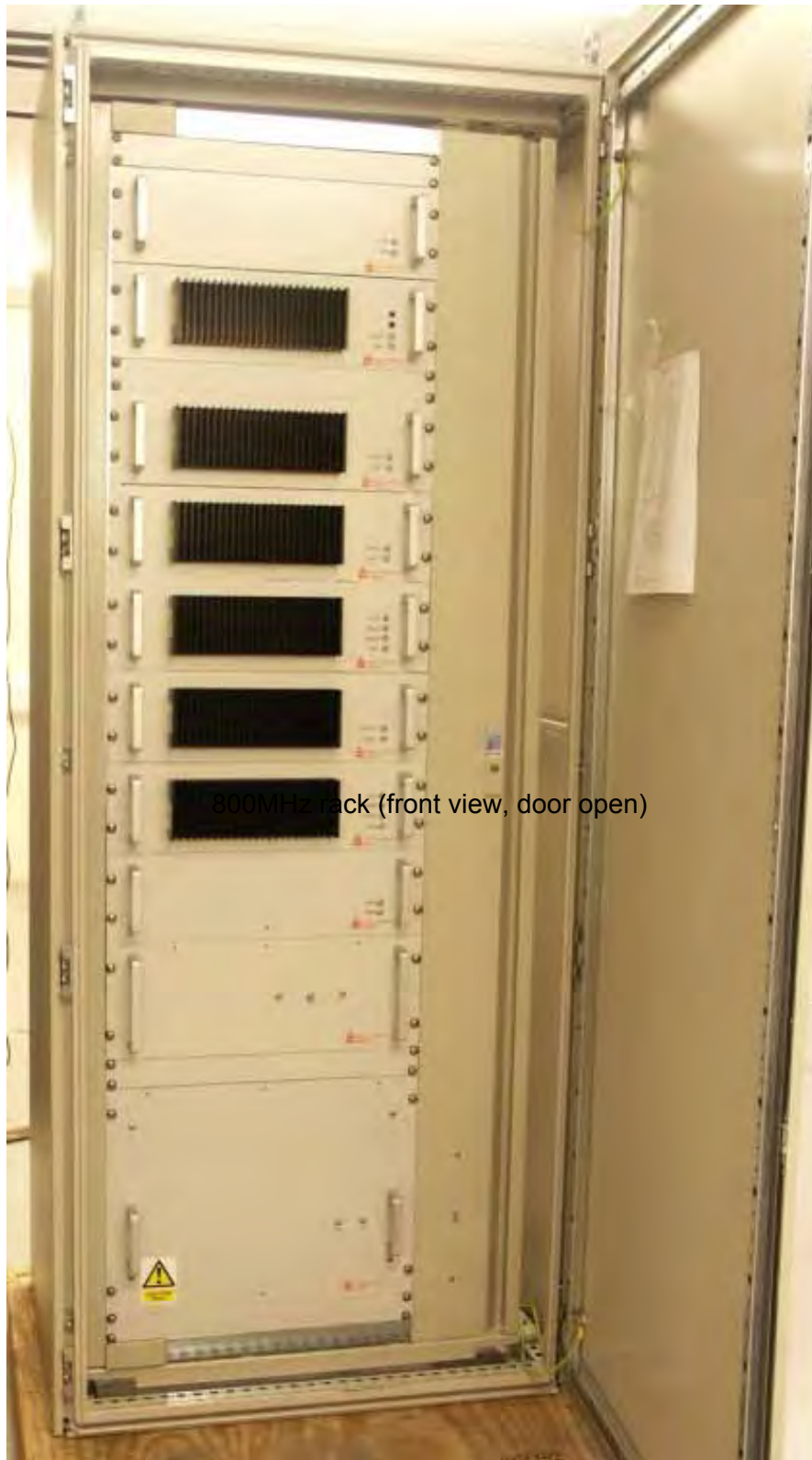
RF distribution rack (front view, door open)
