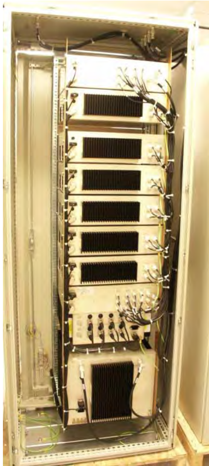
800MHz rack (rear view, door open)
