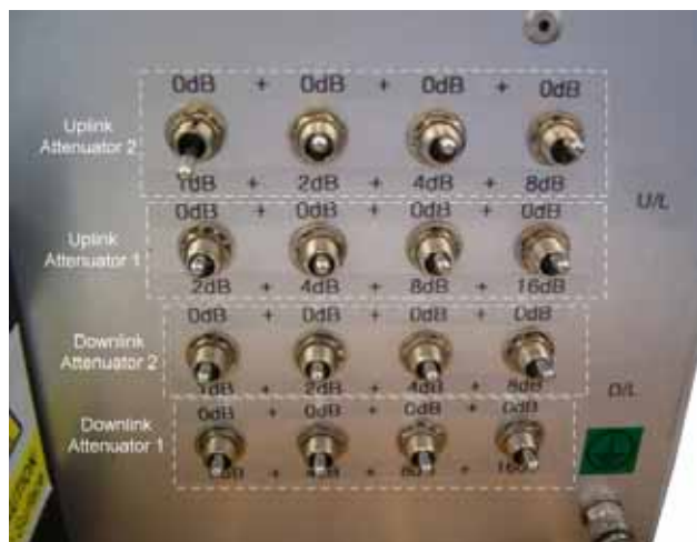
Close-up of attenuator switches
