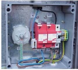
Protective device installed in connection with the power supply
