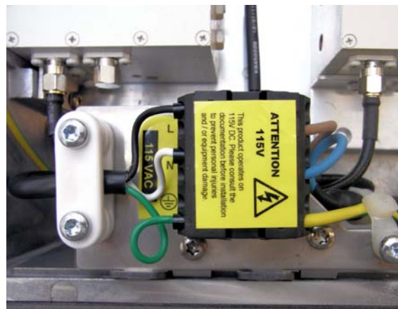
Figure 2-26: 115VAC Power Connections
