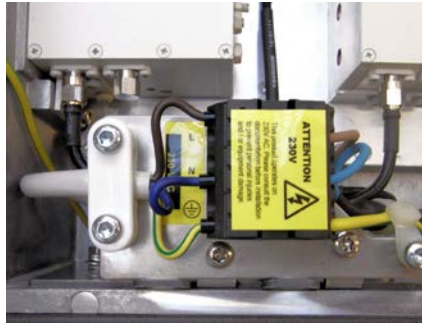
Figure 3-17: 230 VAC Power Connections
