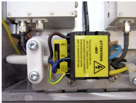
Figure 3-19: -48VDC Power Connections
