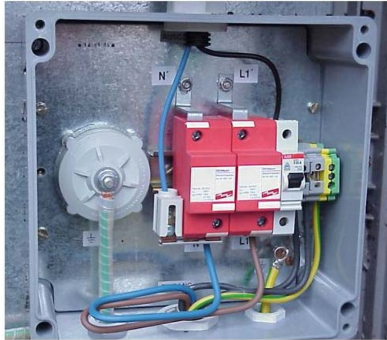
Figure 3-14: Protective device installed in connection with the power supply
