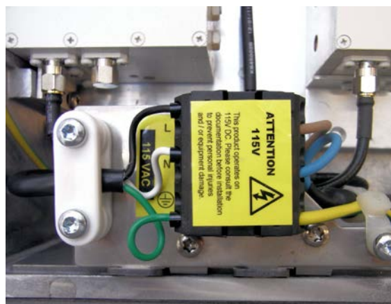
Figure 3-18: 115VAC Power Connections
