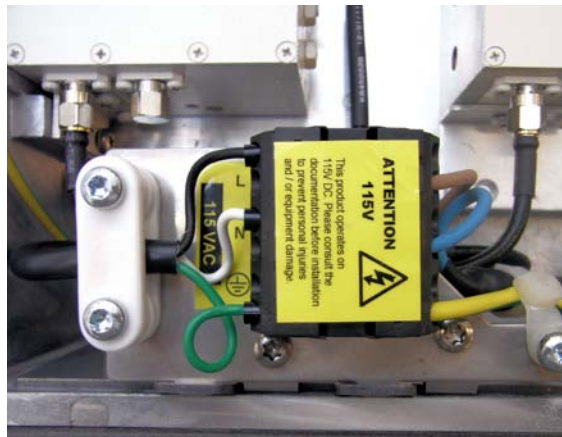
Figure 3-34: 115VAC Power Connections
