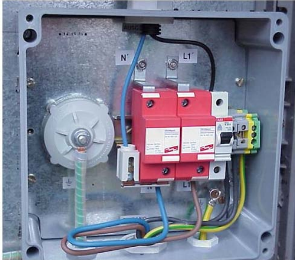
Figure 3-24: Protective device installed in connection with the power supply
