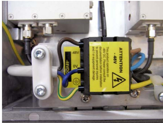
Figure 3-35: -48VDC Power Connections
