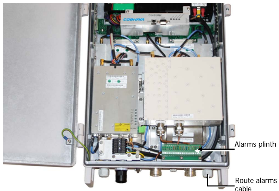
Figure 2-34: Example of Repeater Showing the Location of the Alarms Plinth
