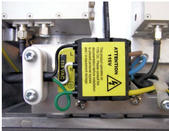
Figure 2-29: 115VAC Power Connections
