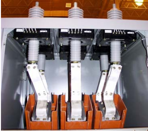
Figure 1. High Voltage Compartment
