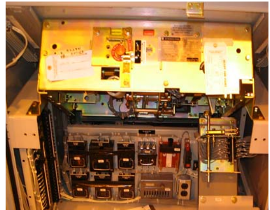
Figure 2. Low Voltage Compartment-Mechanism Side
