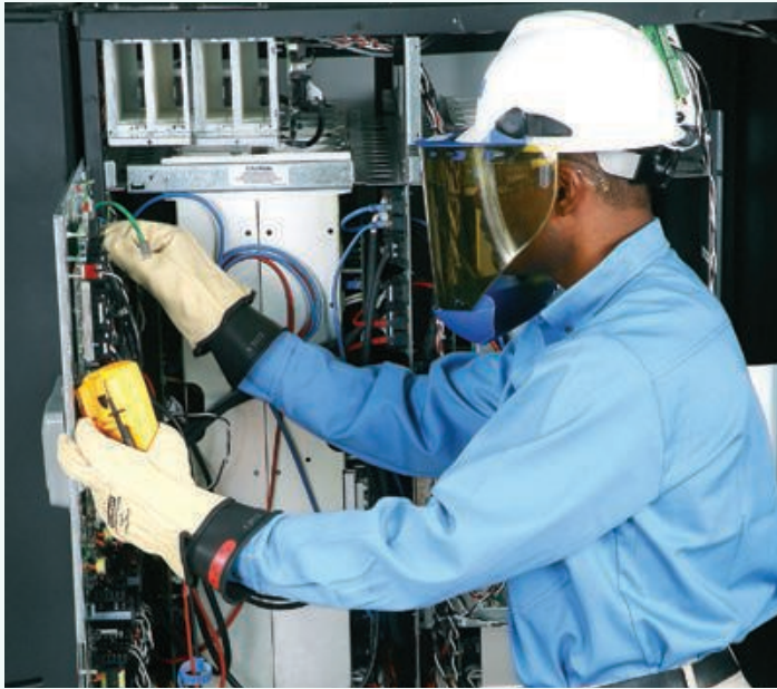
Proper preventive maintenance reduces the risk of UPS failure through thorough inspection, cleaning, testing and calibrating various electronic and mechanical components.
