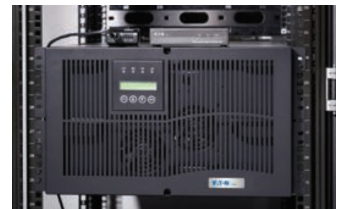
Environmental Monitoring Probe and Environmental Rack Monitor mounted on top of Eaton UPS
