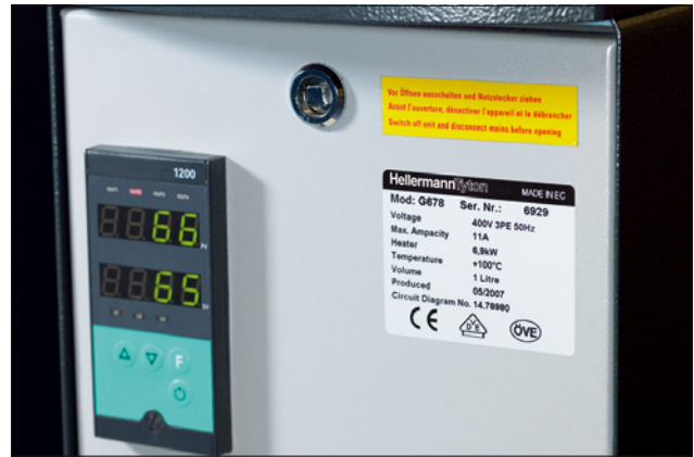
Professional type plate on a heating unit.
