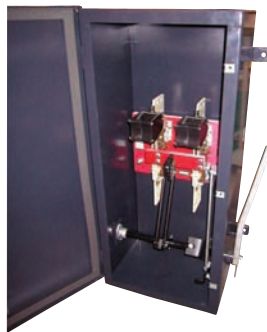
Mill Switch (PMS)
