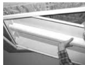
7. *Wire and lay fixture into place by inserting on an angle. For convenience, remove door frame to facilitate easier handling.
