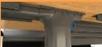
Under Table Cable Management 646
