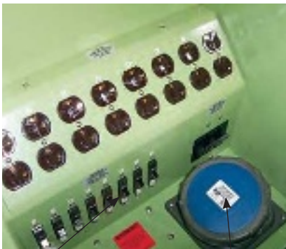
Circuit Breakers (Prewired to Receptacles)
