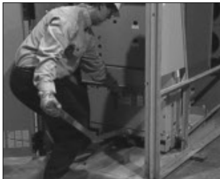
Before: Original floor-mounted lever racking, commonly used on type D and F switchgear, required the operator to stand in front of the breaker with the panel door open.
