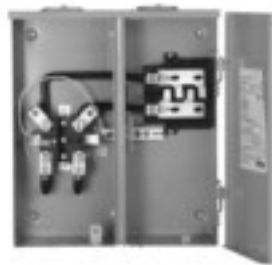
200A meter main (field added), side hinge door
