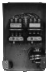
Internal View of NEMA 1 Enclosure Sz 2 2S2W starter with CPT (ESP 100 Overload)
