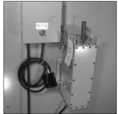
Figure 8 Power and Control switch units.
