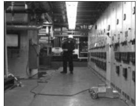
After: Following the field modification, the breaker can be racked in and out while the operator stands outside of the arc flash zone.
