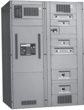
Front View—Circuit Breakers
