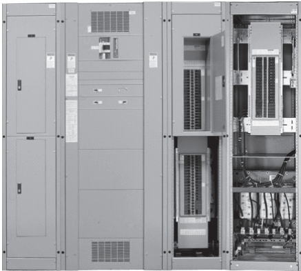
Integrated Facility Switchboard
