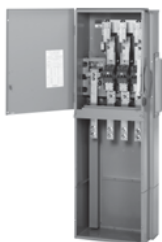
Main Fusible Switch with Utility Pull Box
