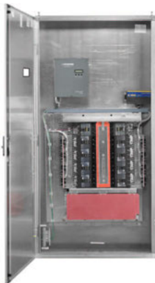
Submetering Integrated Power Center
