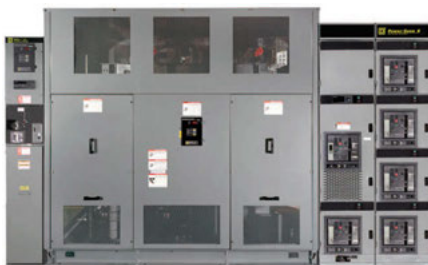
Unit Substation see page 11-17
