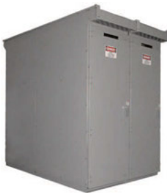
Masterclad 27 kV, Outdoor, Non Walk-in, Metalclad Switchgear
