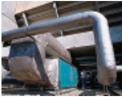
Pumping and ventilation machines
